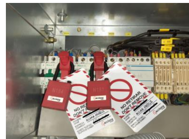
Sistema LOTO instalado LOTO system installed
